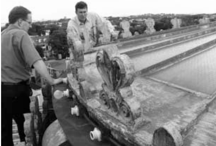
HBI Steeples Project grantee Second Church of Christ, Scientist in Roxbury, MA, gets a roof inspection.
