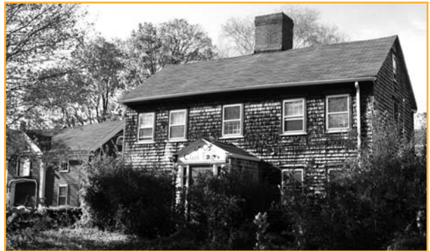
The Federal Period Fowler-Clark Farm in Mattapan was threatened with demolition, but an HBI-funded engineering study proved it was structurally sound and provided support for the Boston Landmarks Commission to landmark the property.
