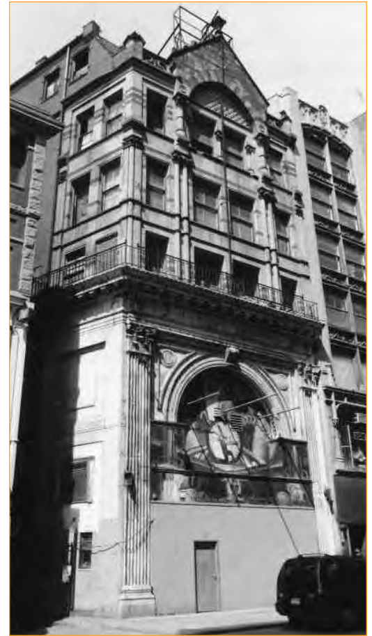
Modern Theater façade as it appears in HBI's 1999 Preservation Revolving Fund Casebook. (Today the façade is covered with protective scaffolding.)
