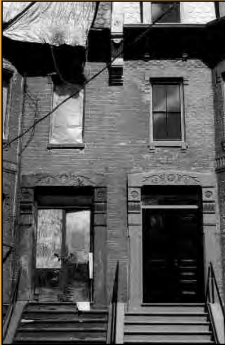
Before and After; Alvah Kittredge Park Row Houses. Photo by Chris Brown
