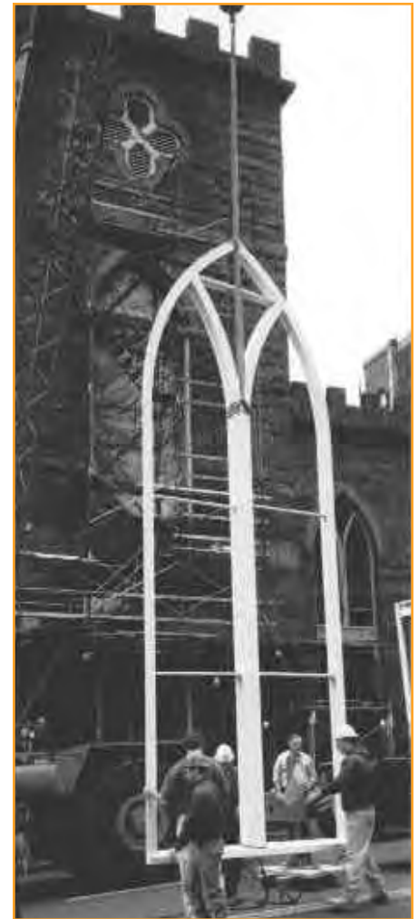
Workers install a newly-fabricated window in the tower at the Church of St. John the Evangelist on Beacon Hill. The wood frame window, funded with help from a 1996 Steeples Project grant, matches the style of others on the facade and replaces a 1960s concrete block style infill of the opening.
